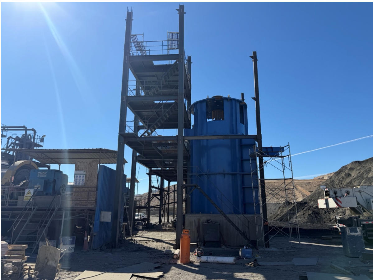
Figure 1: Tower mill, Mariposa Iron Ore Project
