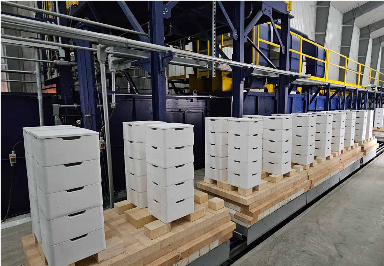
Figure 2.6: Tunnel kiln installed in Calcination Kiln Building
