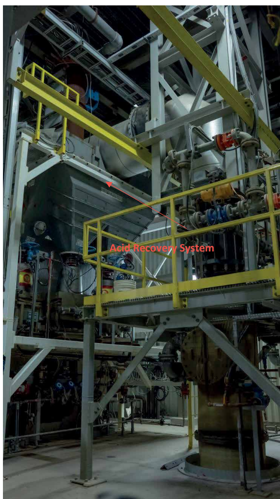
Figure 17. FB01 Feed (ACH) & Acid Recovery Circuit. (Source AEM)
