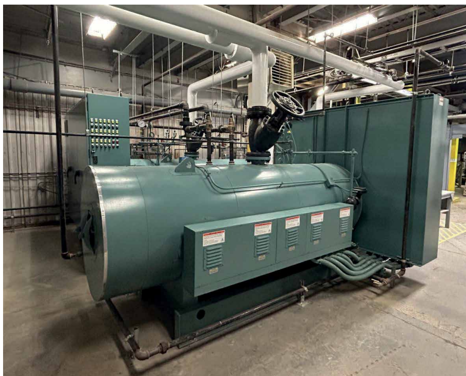
Figure 7. Electric Boilers. (Source: AEM)
