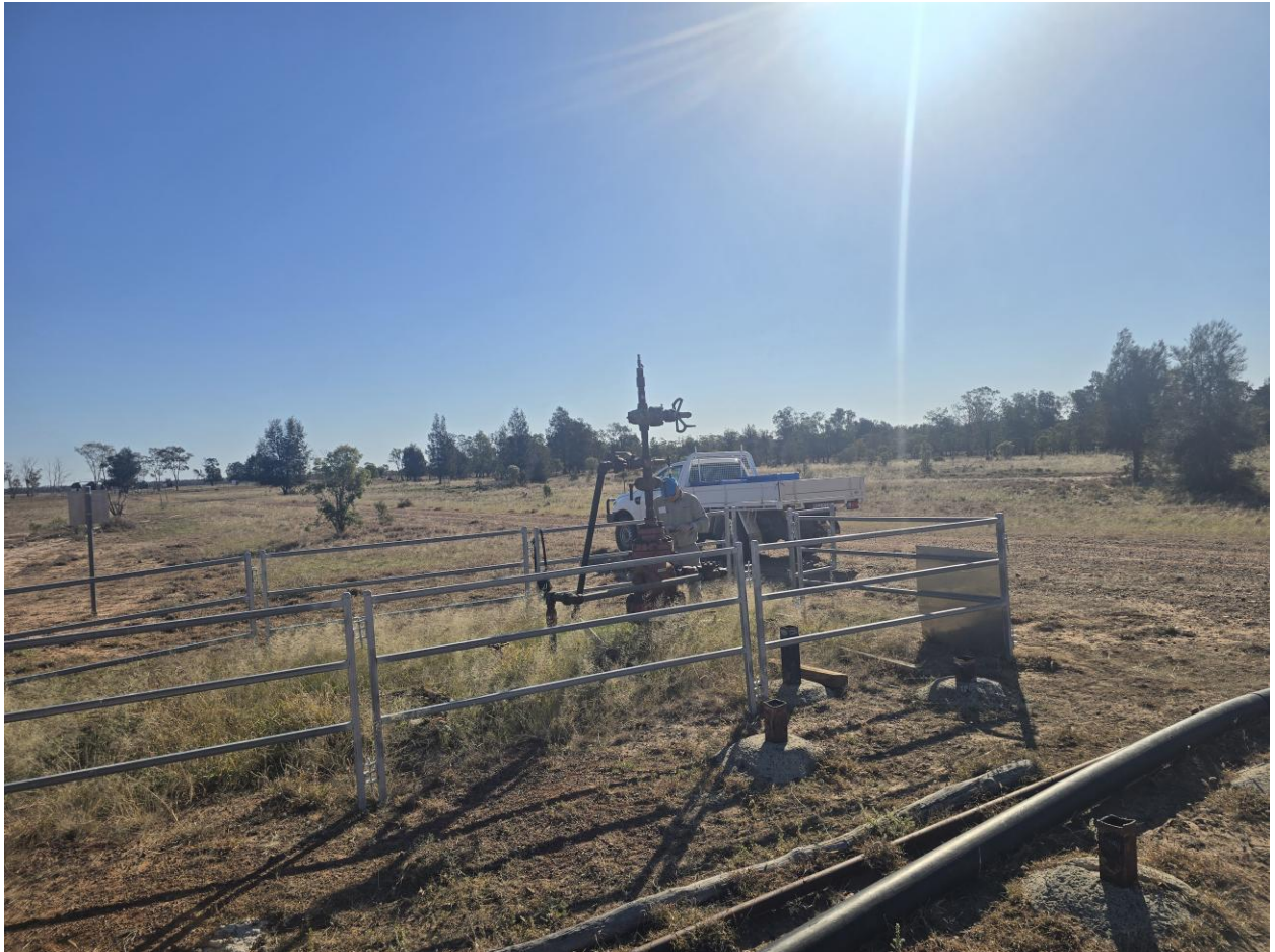
Figure 5 Exploration Manager Len Diekman inspecting Riverslea-3 wellhead as part of plans to free flow the well into the Facility
