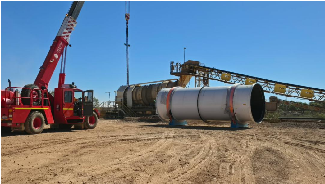
Figure 1. New agglomeration drum delivered to Austral's Mt Kelly Copper Processing Facility.
