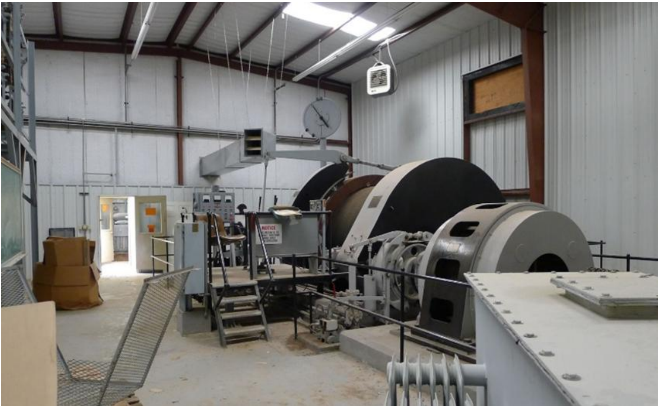
Figure 6: Underground Mine Winch.
