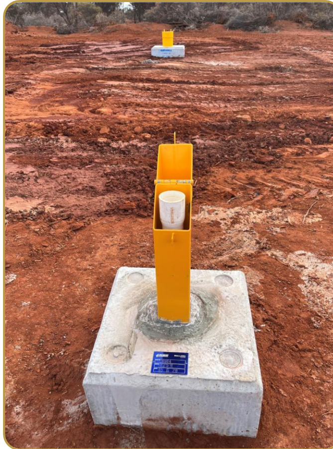
Production bore background and monitoring bore foreground
