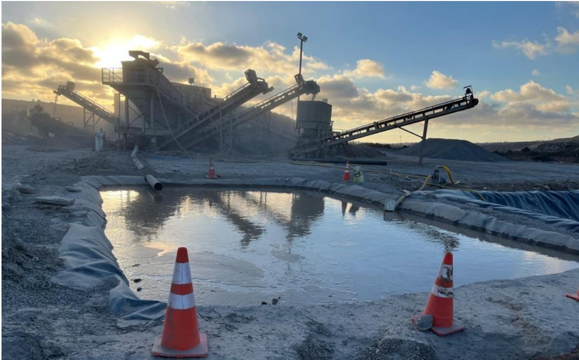
Image 3: Water recycling pools for plant operations
