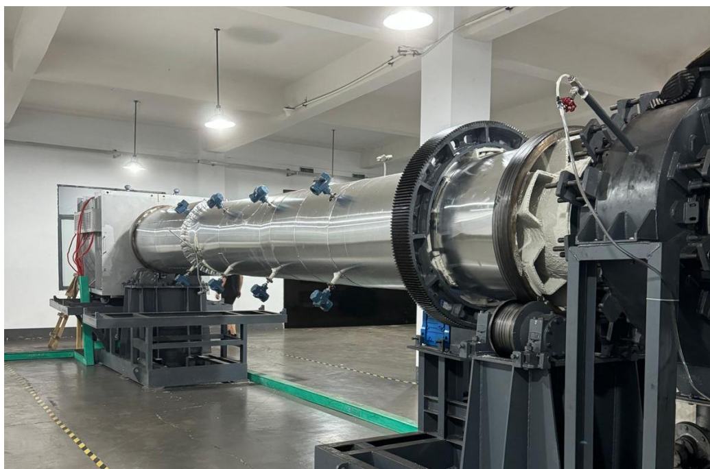
Figure 3: Firebird high efficiency demonstration calcination kiln
