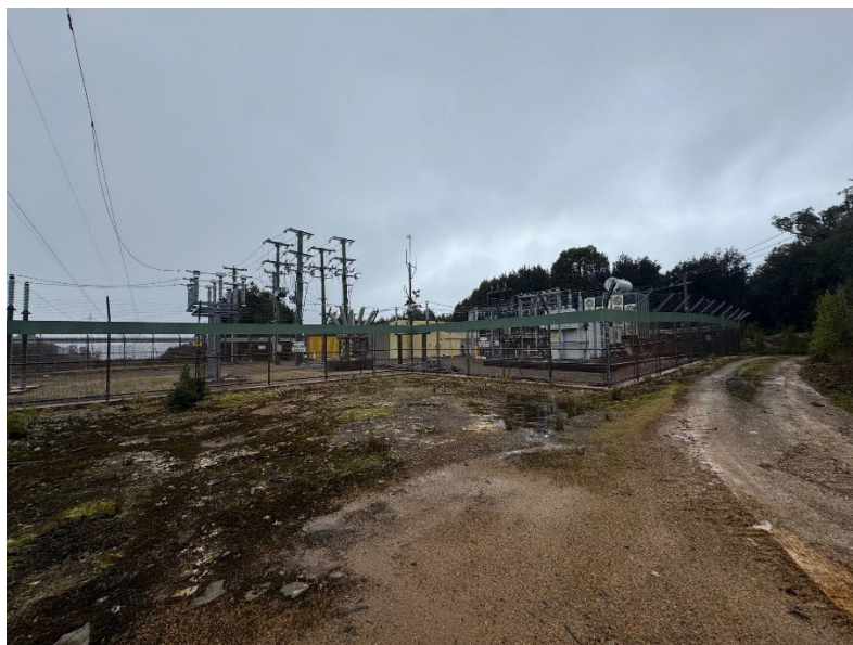
Figure 3 The substation located at Que River
