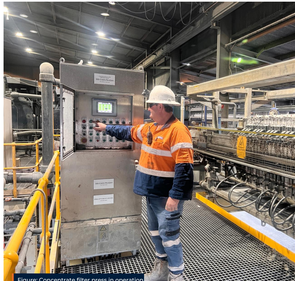
Figure: Concentrate filter press in operation
