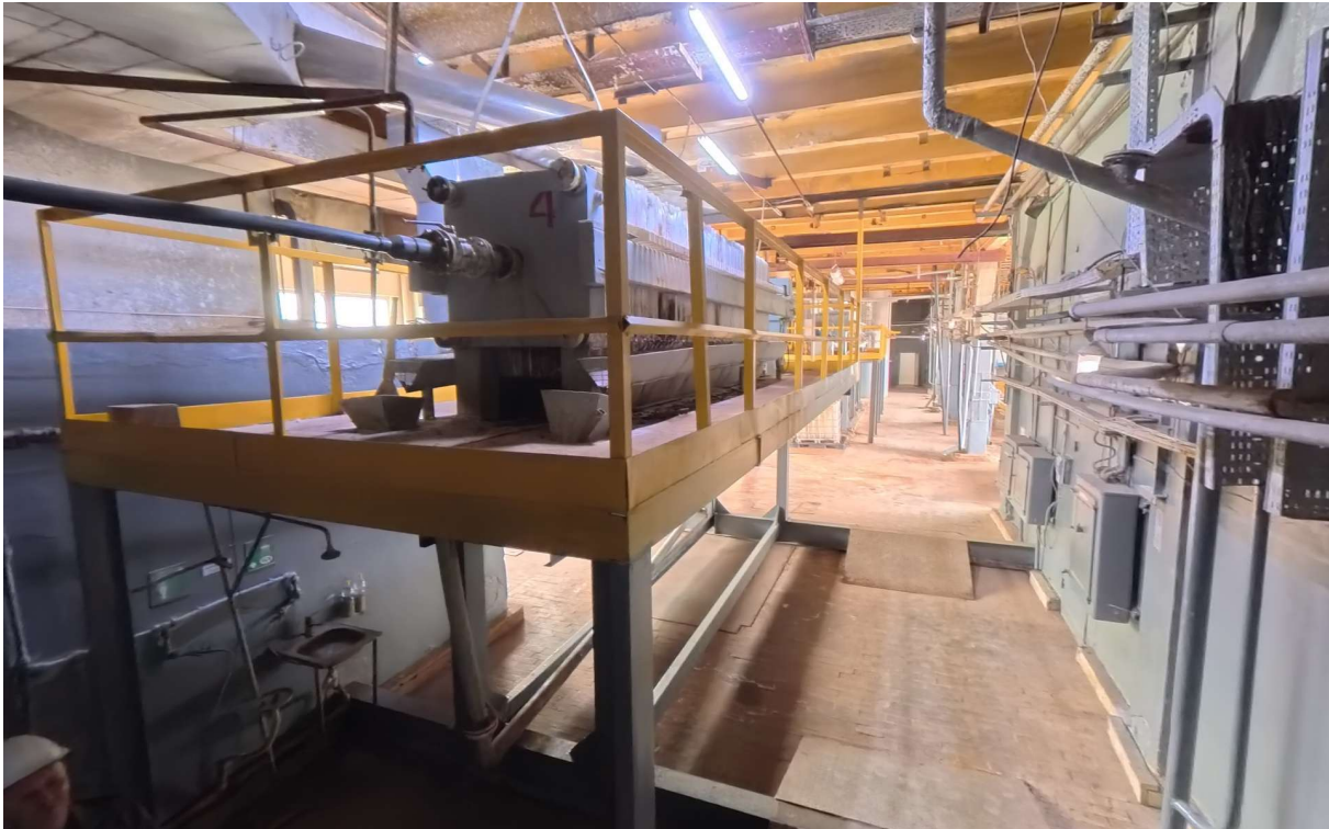
Picture 8. Additional images of the existing infrastructure at the SARECO MREC Facility.
