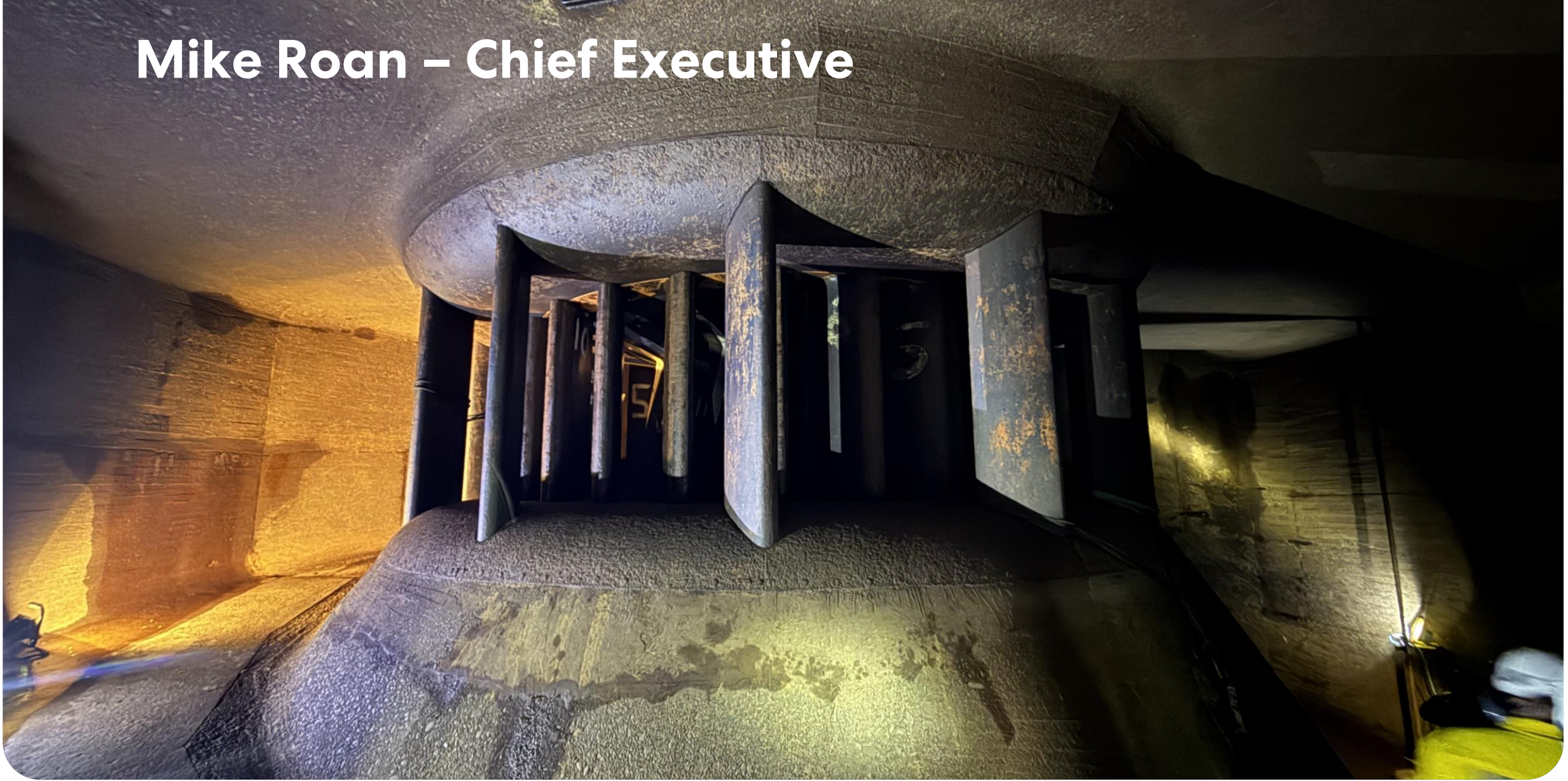
Waitaki Power Station – turbine inlet Unit 6.
