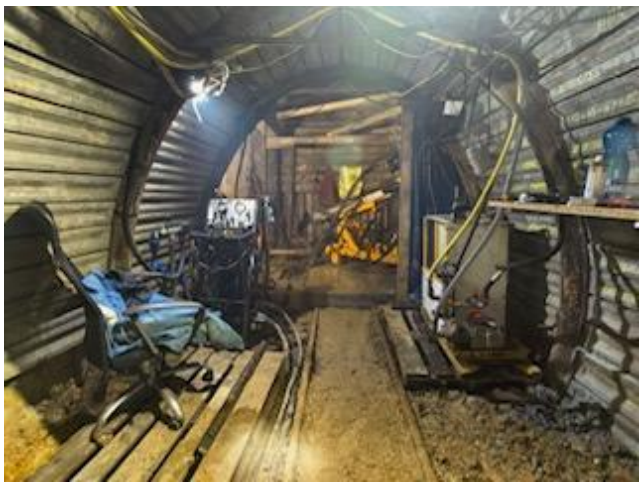
Fig 2: Chamber One fully restored and operational
