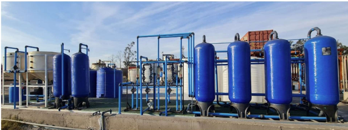
[Figure 2] Example IX plant designed, built and operated by Core IPEX.
