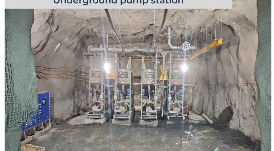
Underground pump station
