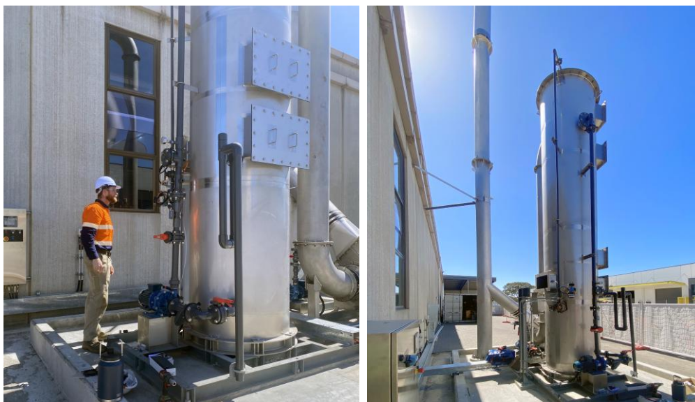
Figure 3. Scrubber at the PSG demonstration facility.
