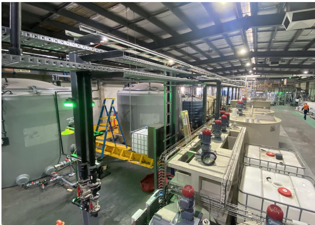
Figure 1. Renascor's PSG Demonstration Facility
