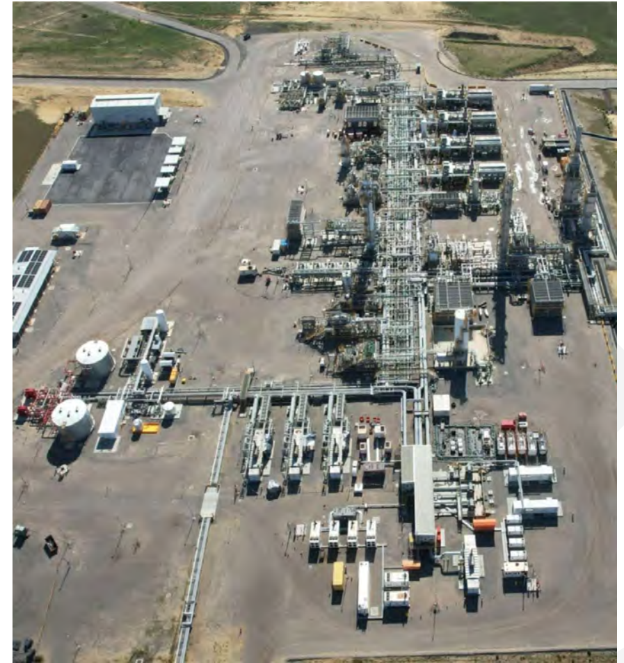
Waitsia Gas Plant
