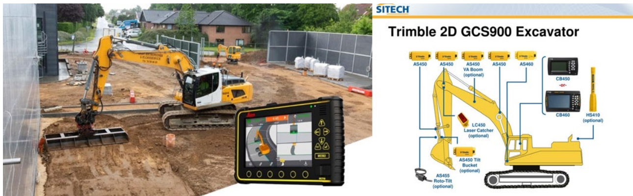
Figure 23: Indicative High-Precision GPS Excavator Machine-Guidance System.
