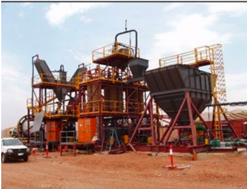
Photo 3: Modular Gravity Plant Installed and operational (as previously operated)
